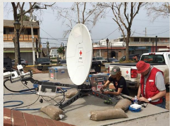
Above) VSAT terminals restoring connectivity in Puerto Rico following Hurricane Maria. (Photo credit: Colin Chaperon for the American Red Cross)
